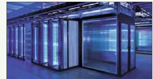
Adamant Data Center Petersburg, Russia, 2012 completed Investor : ADAMANT GROUP Construction Period : 2011 ~ 2012
